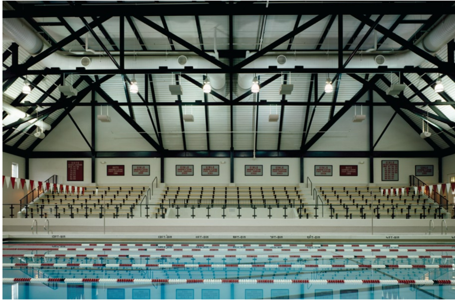
Above: The duct work is woven into the trusses to create a more pleasing aesthetic.
