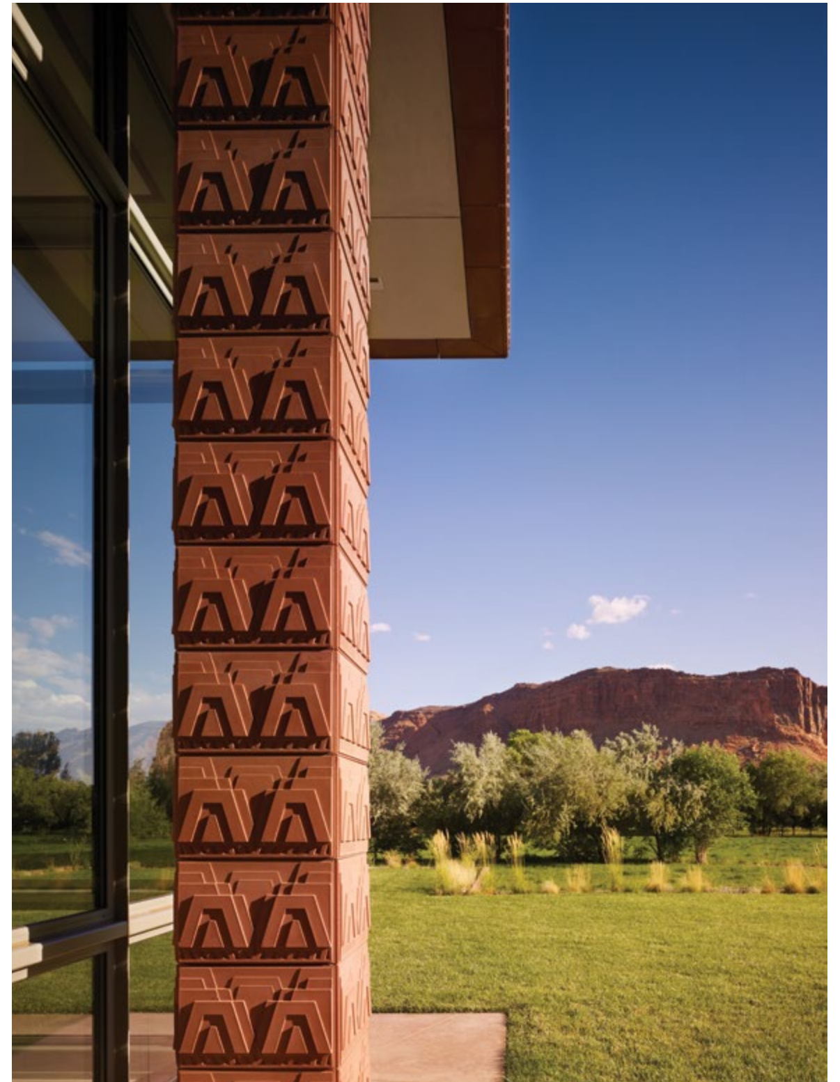
Above: Detail of column supporting living room roof. More than four hundred different shapes of the cast-stone blocks were required.
